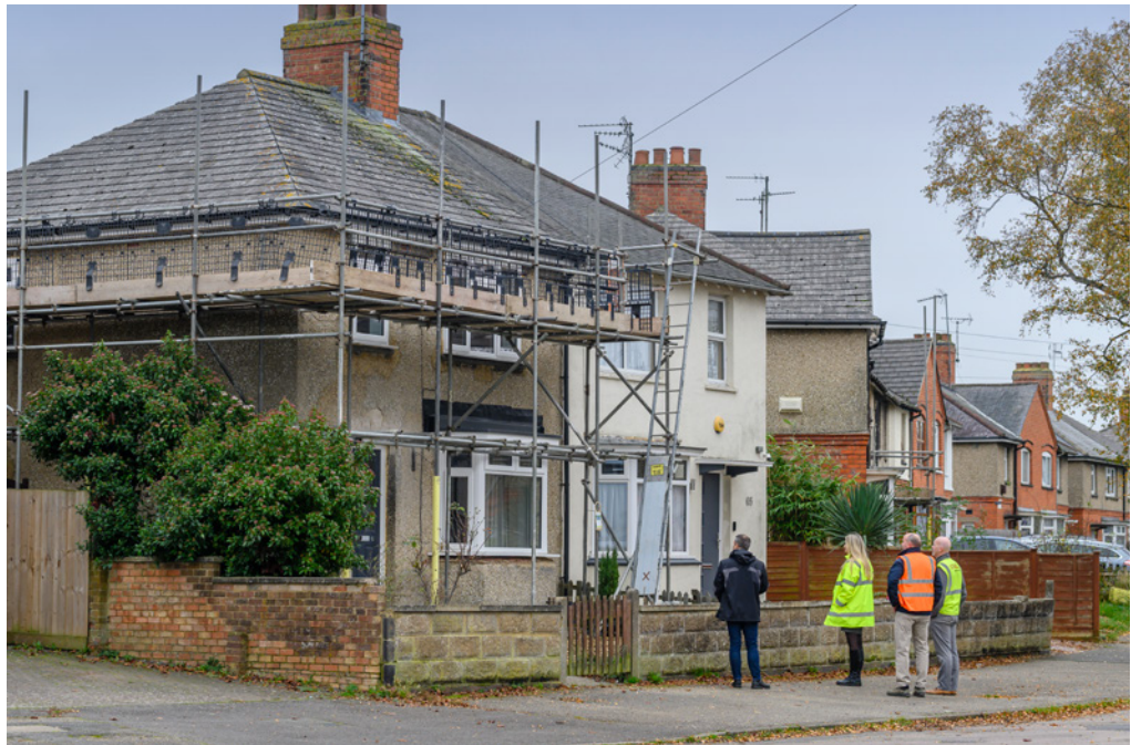
Contractors inspect one of the homes having its energy efficiency improved as part of our Social Housing Decarbonisation Fund project.
